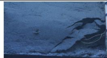
Front Camera, Fracture 3
