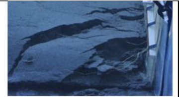
Front Camera, Fracture 4,5,6
