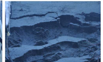
Front Camera, Fracture 11
