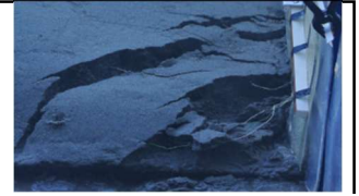
Front Camera, Fracture 4,5,6
